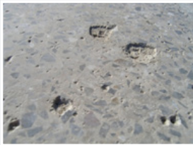
Pop outs in concrete
