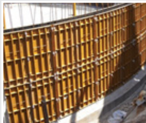
Interim Tank, ONGC, Mumbai, India
