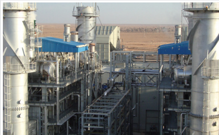
Thermax Boiler Plant, Algeria
